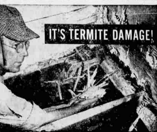
IT'S TERMITE DAMAGE!
