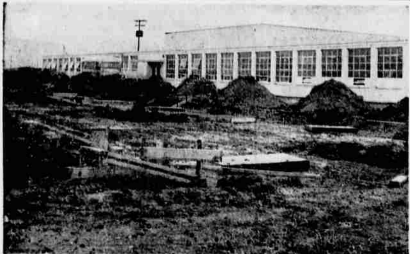
WORK STARTS —Work is getting started on an addition to Jewett school in Central Point as part of school district 6C's building program to provide additional space to re-
