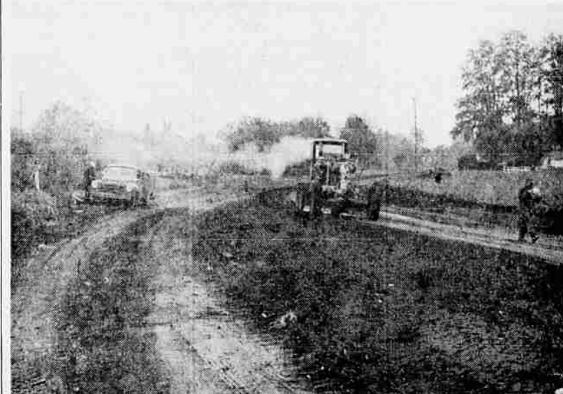
NEW STREET—Work on the section of East 10th st. which will become part of a new thoroughfare between east and west Medford is now at the stage shown above. The streets take a gentle turn to join East 10th st. near Portland ave. The picture was taken looking west, and the Cottage st. bridge is just behind the clump of trees in back of the grader. Paving of the new section will be completed by early fall, but the bridge over Bear creek will not be finished until November, according to Medford Public Works Director Vernon Thorpe.
