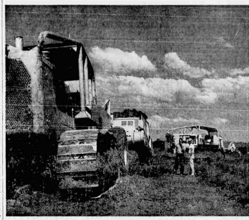
LEVELING —C. C. Hoover and his sons are leveling a thousand acres in the White City area partially for subdivision development and some for agricultural purposes. Shown inspecting their work are heavy equipment operators Glen Nelson, White City (with the cap), and Wally West, Central Point. Both men work for Steve Wilson, contractor for the job. The picture was taken recently at the 400-acre tract on Antelope rd. The hardpan ground is being ripped up during the leveling operation.
