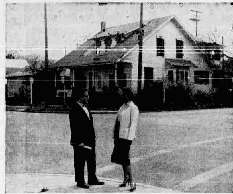
BUILDING SITE —The new building for the Medford chamber of commerce will be located on the site now occupied by the two story frame house above, on the corner of 10th st. and Riverside ave. Dismantling of the house is now under way. Tony Manno, of Acme Hardware co., is shown chatting with Chamber Secretary Mrs. E. S. Boyd in front of his place of business. Detailed plans for the new structure are expected to be revealed in about a week, according to Chamber Secretary Don McNeil.
