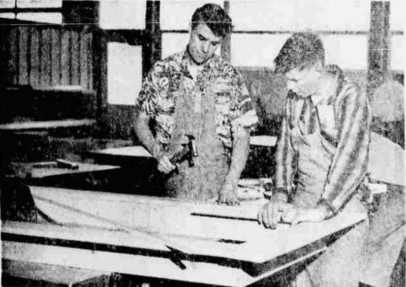
CARPENTERS — Working on door frame that is part of a good-sized prefabricated building being built in the Medford High school wood working shop, student Barry Holt hammers while Everett Musie keeps the corner square. All phases of wood working, from construction to applying finish, are taught.
