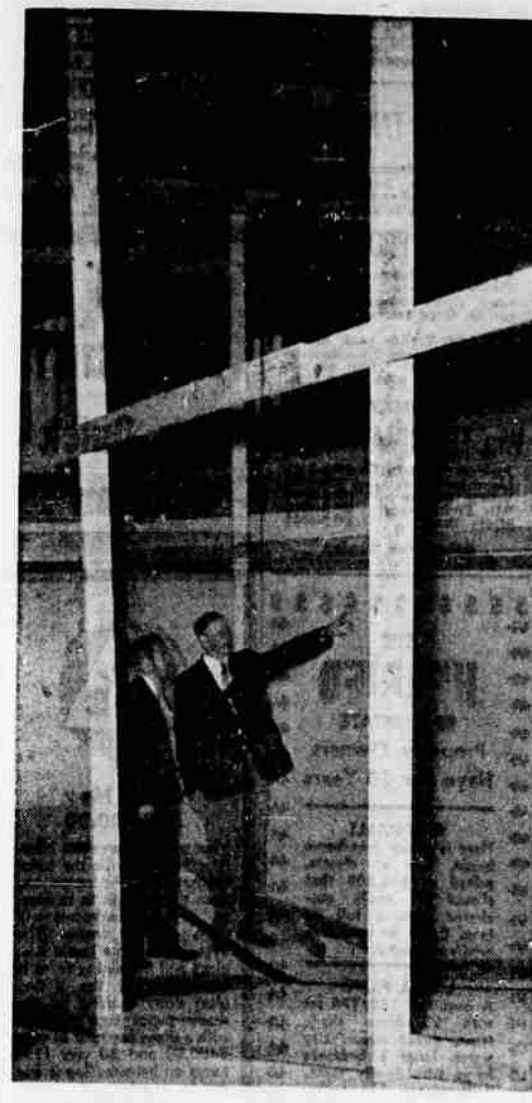
CHECK POOL —Robert L. (Bob) Jones, right, secretary of the Medford YMCA, and Dave Curzon, physical director, check the deeper end of the swimming pool at the YMCA during renovation. The pool was repainted, and other work was done in the room housing the pool. Jones said the pool reopened yesterday. (Reid Witter Photo)
