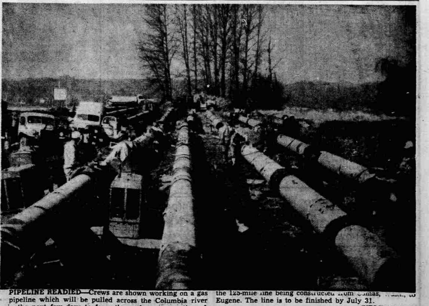
PIPELINE READY —Crews are shown working on a gas pipeline which will be pulled across the Columbia river in the next few days to form the underwater portion of the 125-mile line being constructed from Canas, Eugene. The line is to be finished by July 31. (UPI Telephoto)
