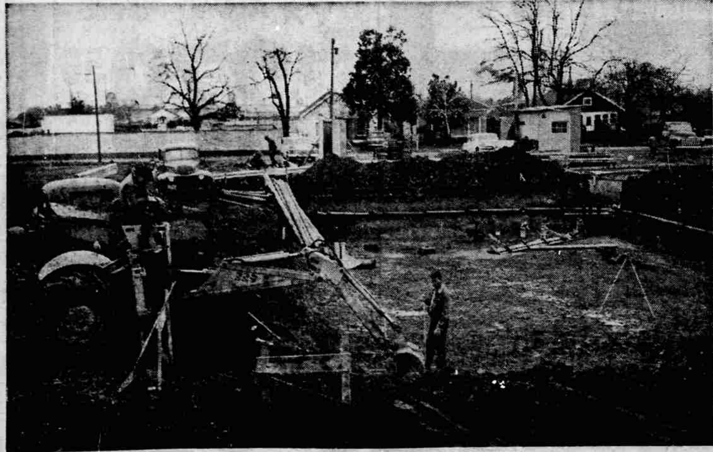
SWIMMING POOL SITE - The $85,000 Jackson park swimming pool project, tentatively scheduled for completion by early May, is now 40 per cent complete.
