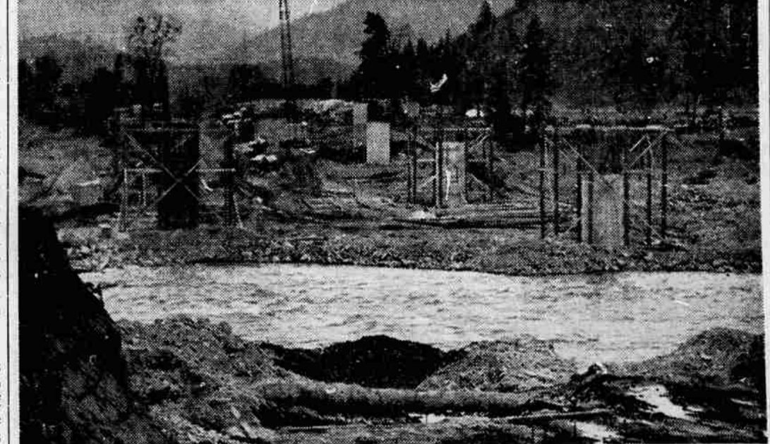
BRIDGE SITE — Rows of giant piers that will support the new Highway 99 freeway bridge over the Rogue river, loom up from the river bank in the vicinity of Homestead on the Rogue. The bridge is the dividing point between the Evans creek-Homestead section and the Homestead-Rock Point section, both of which are currently under construction. Grading of both sections is expected to be completed this fall. According to construction engineer Al Chapman, the bridge will consist of two separate sections, two lanes for northbound and two for southbound traffic. The structure, including approaches, will total nearly 600 feet in length.
