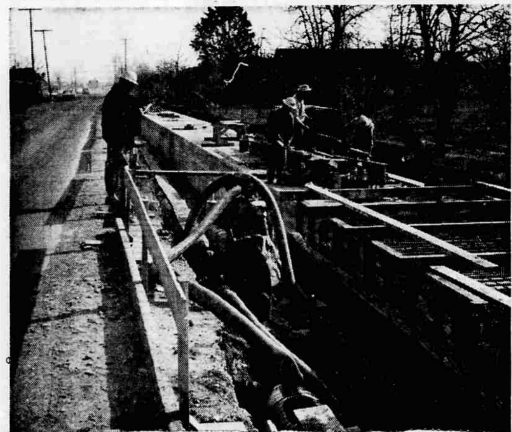
CONSTRUCT CULVERT —The second of a four by eight foot concrete culvert, that will eventually extend from the Southern Pacific tracks to Kings highway along Stewart ave., is now under construction by county crews. The first section, 430 feet long, was built last year. The one under construction will reach 700 feet to the Holly st. intersection, and two more sections will be built in succeeding years, according to County Engineer Robert Carstensen. The culvert will replace the large ditch that serves as a drainage canal for the Kings highway area, and will make it possible to widen Stewart ave. The county owns the south half of Stewart ave. in this section and the city of Medford the north half. County Bridge Superintendent Wesley Hartman, left above, checks on the construction progress.
