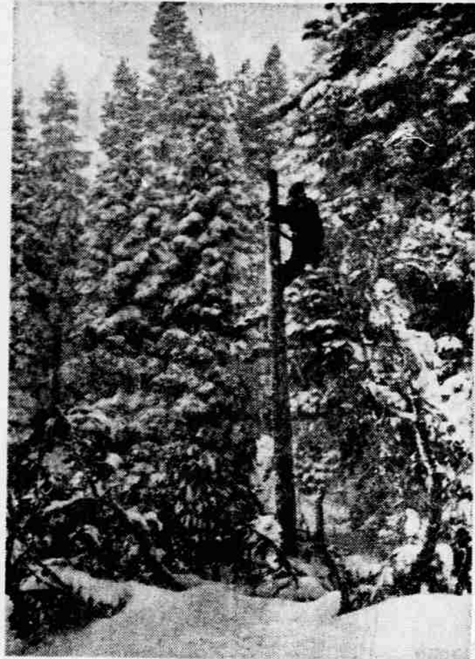
DAMAGE REPAIRED —Downed telephone lines are being repaired at Squaw Valley, Calif., by telephone repair teams after two days of gale winds and rain—topped by a raging blizzard, took their toll. Einar Nelson, on pole, and Bob Cannon are almost undistinguishable by the heavy snowfall as they make repairs. (UPI Telephoto)
