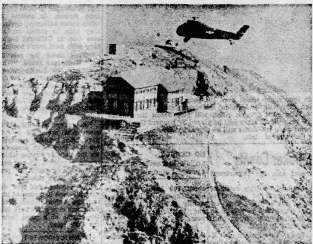
LOWERS SUPPLY —A U.S. Army helicopter hovers above the lodge at the summit of Italy's Mt. Grignon after lowering a supply of building material to workmen on the peak. The aluminum and glass chapel is being erected by members of the Alpine club of Milan as a memorial to climbers who have lost their lives on Mt. Grignon. (UPI Telephoto)
