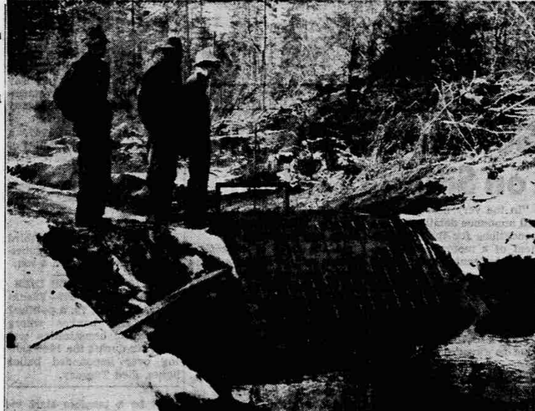
INSPECT STRUCTURE - T. C. Cunningham and Dave Neville of the Nye Ditch Users, Inc., and Robert Lonsway, of the Sams Valley-Beagle Soil Conservation district, stand at the intake structure where a new concrete ditch takes water from Mill creek.
