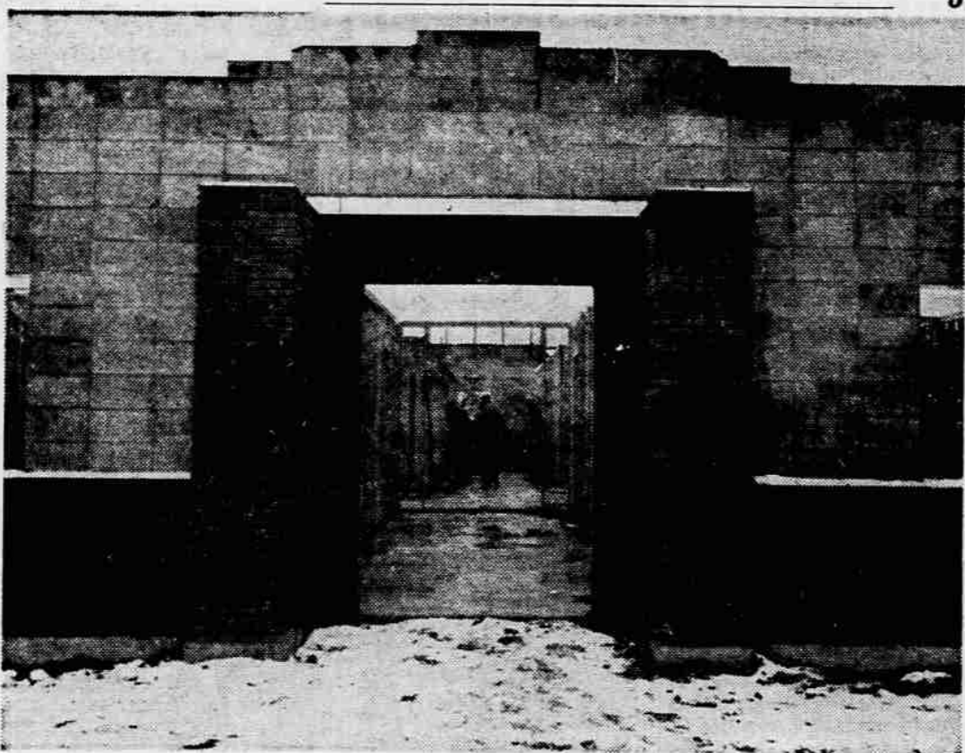
HOSPITAL ENTRANCE — The front entrance to the new Osteopathic hospital in Central Point, currently under construction, was at this stage of completion last week as plumbing and some carpenter work went on in spite of ice and snow. All the exterior walls of the building are up, with construction going pretty much on schedule, according to Medical Director Dr. Paul T. Rutter. Completion date will be about May 15, Dr. Rutter said. The city of Central Point has extended Second st. to the hospital property line and water and sewer facilities have also been provided.
