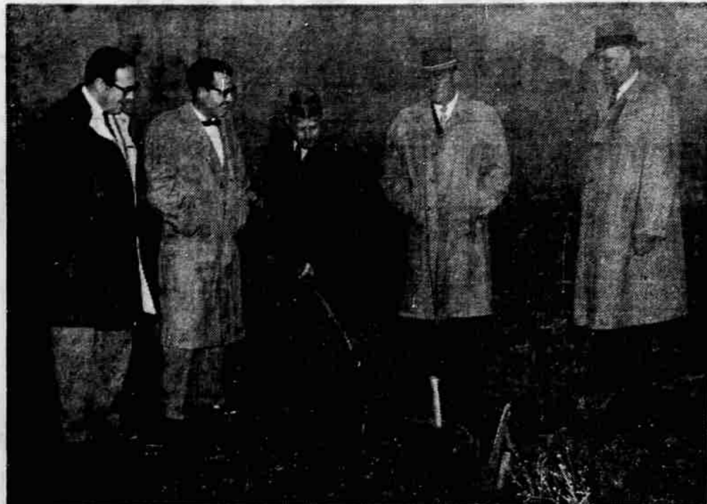
BREAK GROUND —Councilman Robert Van Sickle takes the first shovelful of dirt from the site of the Jackson park swimming pools. Watching him with obvious satisfaction that the project is finally underway are, from left to right, Robert Haworth, city parks and recreation director, Russ Jamison, president of the parks and recreation commission, Robert Bacus, city councilman, and Mark Goldy, representing the Jackson County Housing Authority. —(Knackstedt Photo)
