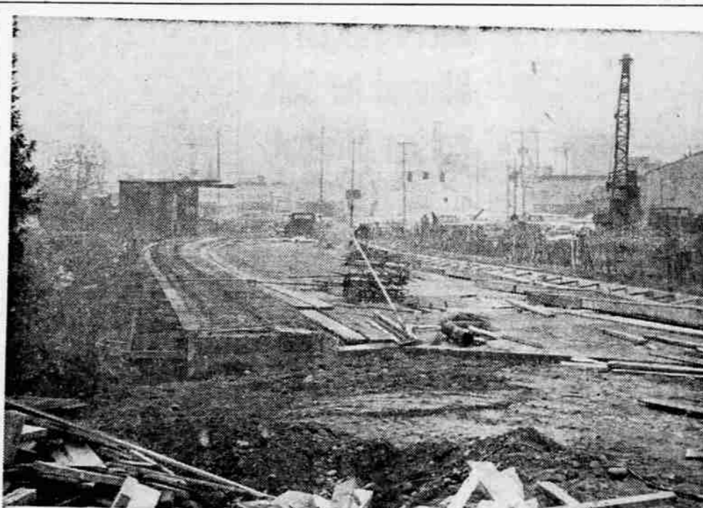
NEARS COMPLETION — The Eighth st. bridge over Bear creek started looking like a bridge late last week as the concrete for the deck was poured. Earlier pouring was delayed by cold temperatures. The concrete will not be hard enough to permit vehicles to use it until January it was reported. Work is progressing on the sidewalks and railings.
