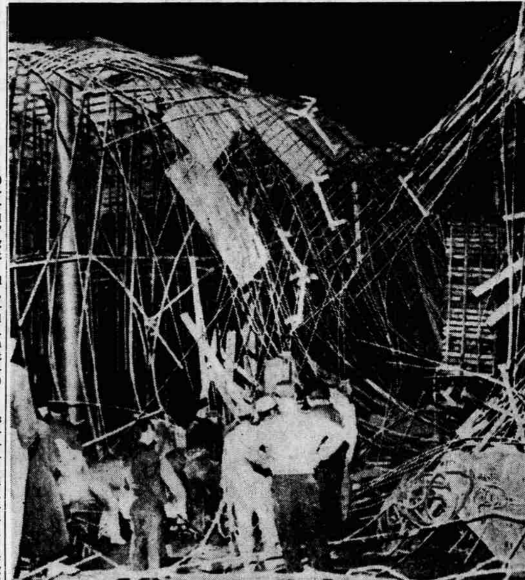
SEEK BODIES - Rescue teams Friday in the east end of Montreal, Canada. Three searched for bodies of workmen killed when men were killed, one was missing and 20 an almost completed factory roof collapsed were reported injured. (UPI Telephoto)
