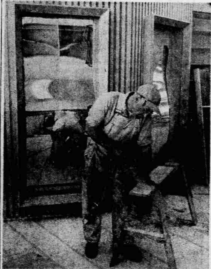
PREPARE FOR OPENING - Carpenter Clyde Richmond, Medford, is preparing finish work in Gallenkamps shoe store in the Medford Shopping Center. The shoe store expects to open sometime next month, and will be one of many in the development. Other stores opened Friday, while some opened earlier. Richmond is employed by Fixture Contractor Berg Kalmer.
