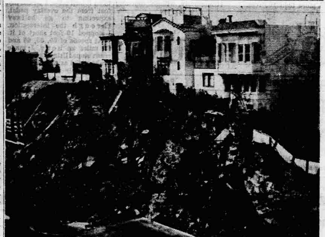
EVACUATED BY SLIDE —Residents of five duplex apartment houses were evacuated after a landslide at the site of a 16-story apartment building excavation in San Francisco. Soil and structural engineers are conferring on methods to prevent further slides and make the five buildings safe, as well as accessible. (UPI Telephoto)
