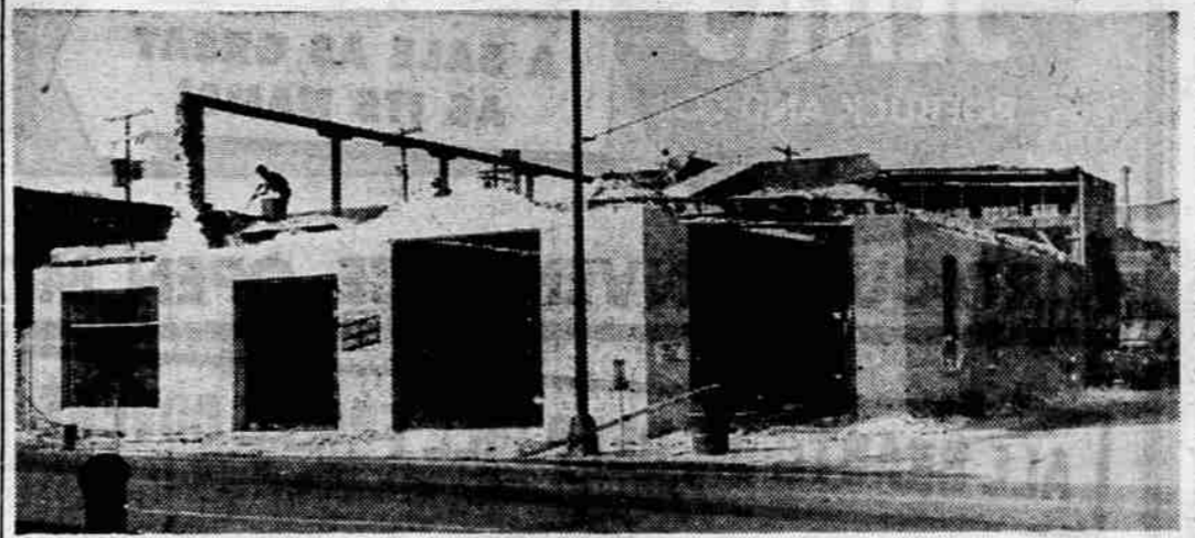
UNDER CONSTRUCTION—This picture, a view from Riverside ave. to Bartlett st., shows Daly's garage being torn down. This is the newest of the parking lots in the
