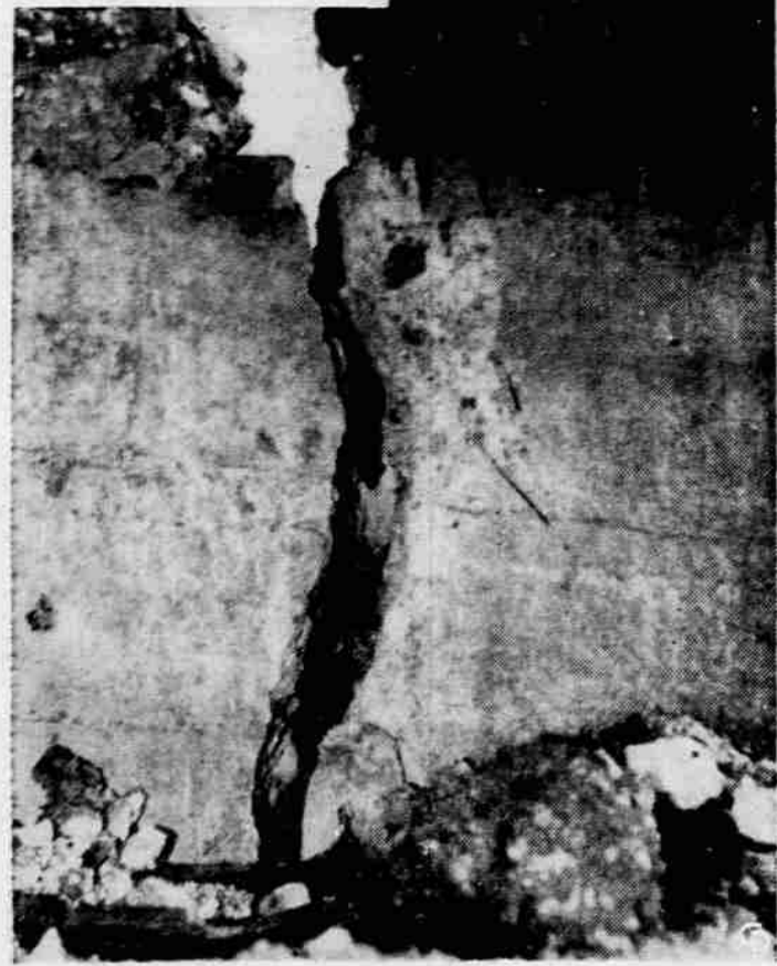
CRACKED WIDE OPEN and under 24 hour watch Hebgen Dam in Montana shows the earthquake ravages to the core of the dam. Officials fear another shock might split the dam even more, causing water to break through.
