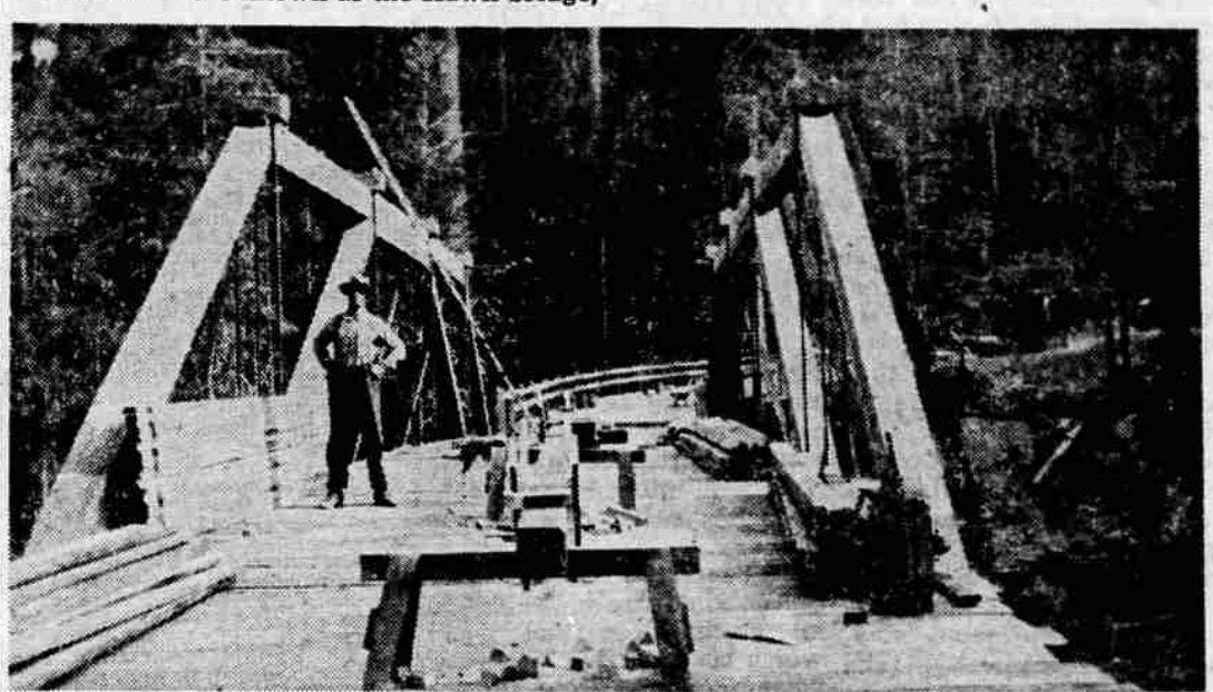
UNDER CONSTRUCTION —This picture of the Hawk bridge over Big Butte creek was taken by Wesley Hartman before the "cover" was put on. Man in the picture is his brother, Lyal. The Hartmans had a box camera with which they took a great many pictures of bridge construction during the 1920's. All except two of the pictures here are from their photo album.
