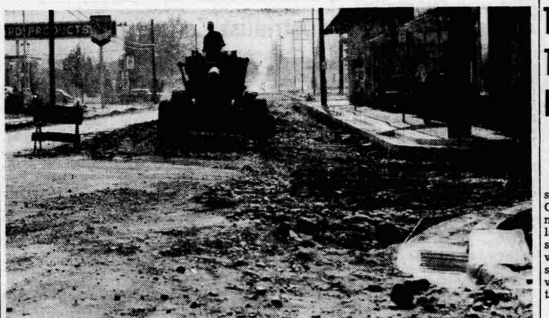
DOWN TO EARTH—Work progressed this week on the widening and paving of East Jackson st. from Bear creek to Genessee st. Tru-Mix Concrete company for a sum of $25,254.85. This view, westward from Genessee, shows a grader working in front of the B and G
