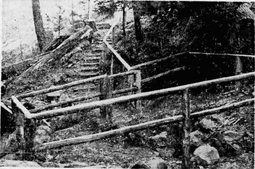
SPRING ENCLOSURE - McCallister soda springs site, which for years has been uncared for, was recently made into a first class camp area by the forest service and the spring itself was enclosed with a fence
