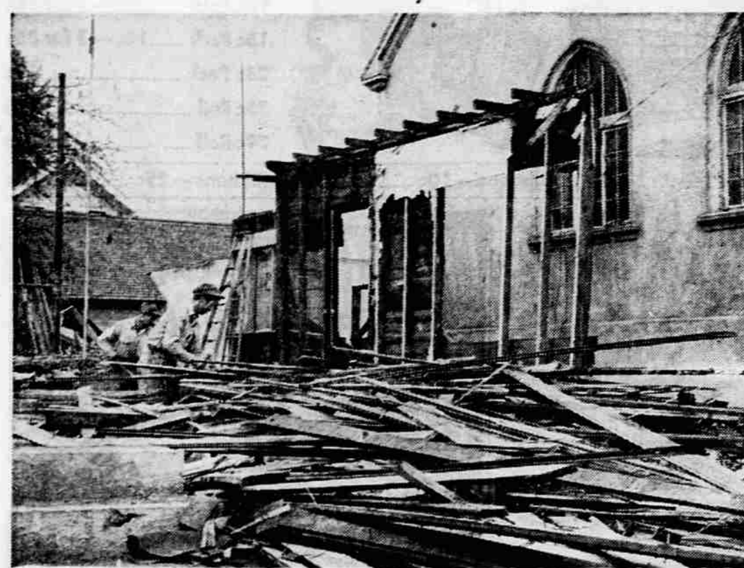
CONSTRUCTION PROGRAM - Work was started several weeks ago on the clearing of property near Zion Lutheran church, Fourth st. and Oakdale ave., for the construction of a new $95,000 Sunday school building. Razed was the former primary building and two other Sunday school buildings will be torn down in February. Two workmen, Elmer Denzer, Phoenix (left), and Lyle McGinnis, Dark Hollow rd., employees of Gordon Logan, contractor, work among the rubble of boards from the old building. The church building is at right.
