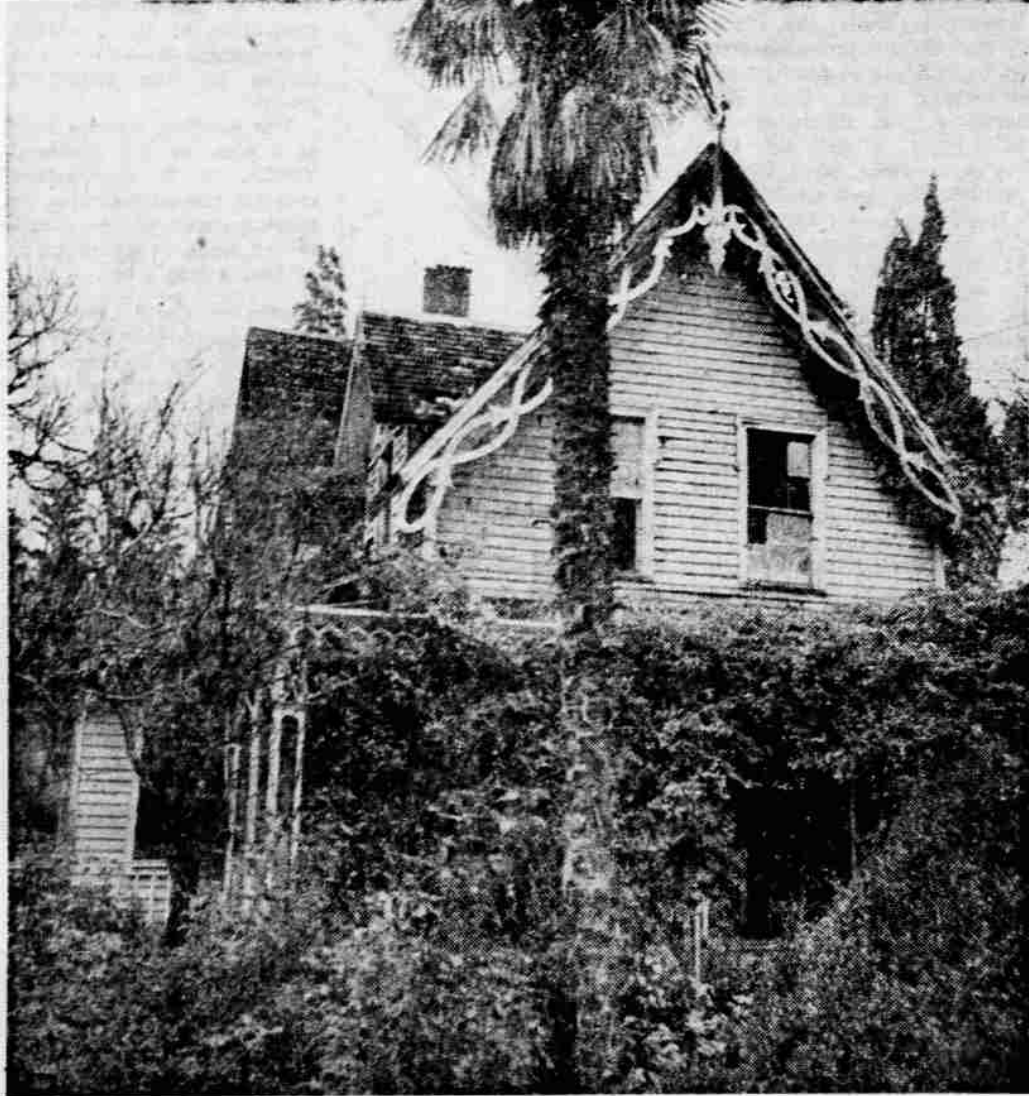
BRITT HOME —Here is the historic residence itself, one of Jacksonville's landmarks. Broken windows on the second floor and an un-
