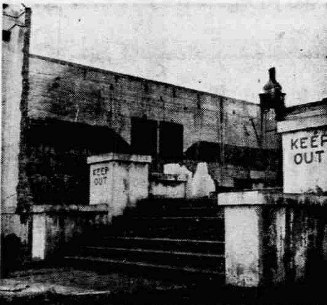
RACK AND RUIN? —The old armory building is certainly well on the way. Back around Halloween, some young vandals wandered through the hallways and rooms in the front of the building, breaking windows, kicking out chunks of plaster from the walls and painting obscenities. Fire was the main culprit in 1951. Replacing this massive relic with a modern structure, needless to say, is a major enterprise. Even demolishing it and turning the lot into a park or off-street parking area is a big order. Nevertheless, as it stands now it is one of Medford's prime eyesores—and a danger to children.
