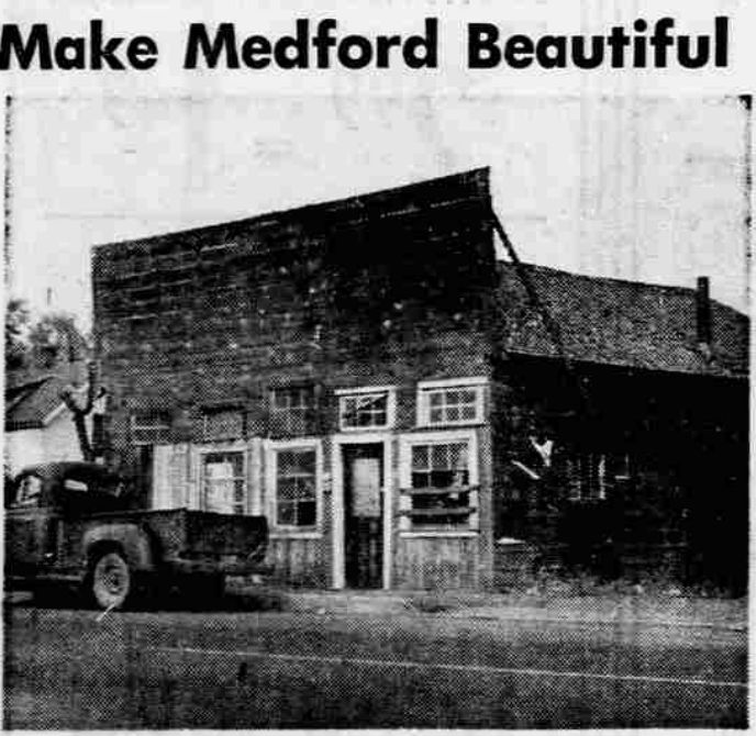
WILD WEST—This building would look more suitable in a TV western than on a main thoroughfare in Medford. It needs a coat of paint and some new windows, to say the least. This picture is another in the Mail Tribune's inventory of eyesores which could be rectified to help "Make Medford Beautiful."
