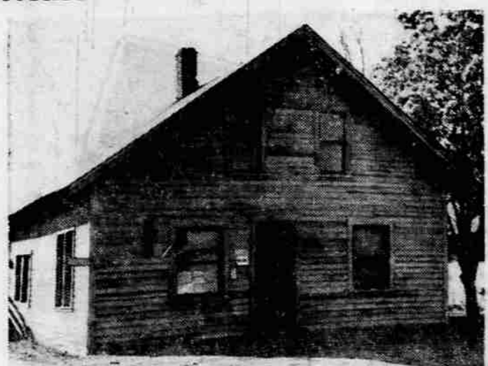
DILAPIDATED —A number of buildings in varying states of disrepair line Medford's north-south thoroughfares. This particular structure with its tiny "For Sale" sign by the door is sagging, needs paint. Improving its appearance would help sell it—and help sell visitors on Medford. This scene is one of a series appearing in connection with the city's "Make Medford Beautiful" campaign.
