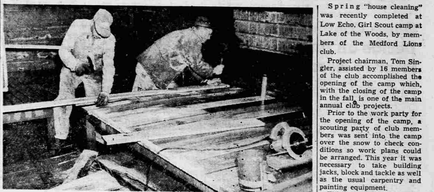
CARPENTRY WORK—Tony Capello (left) and Jim Dziarmaga rebuild a porch on one of the buildings at the Girl Scout camp at Lake of the Woods during the recent work day at the camp by members of Medford Lions club.
