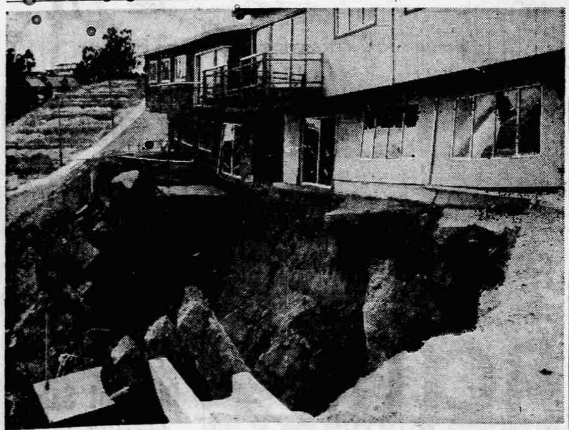
ON THEIR WAY—Two new homes in Oakland, Calif., constructed on filled land, are moving down a 100-foot slope toward the road at left. The houses' 20-foot patios, which have already dropped away, had been supported by the concrete pilings here shown leaning over to the left. The houses have been evacuated, all utilities cut off and a large trench has been bulldozed at the bottom of the slope to catch the houses and dirt before they reach the road.
