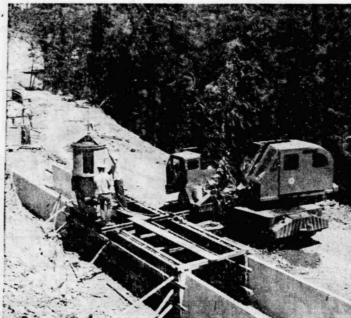
CONCRETE PLANT —A portable plant mixes concrete on a construction site at the Talent project. This is one of four such plants. Small rock is mixed with sand in the section to the right of the picture. This is carried on a conveyor belt to the cement silo on the left. The cement pours from the silo along with the rock and sand into a hopper which in turn pours into the cement mixer truck.
