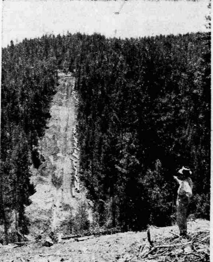
CLEARING FOR SIPHON —James Callan, project engineer in charge of the Talent project for the bureau of reclamation, points to a strip of clearing through heavy forestation. Through this strip of bared ground the Soda Creek siphon will be installed. Pipe for the siphon are shown alongside a ditch. The half-mile long siphon will connect two canals. Not shown is the canal just beyond the trees which will help transport water to the Green Springs power plant.
