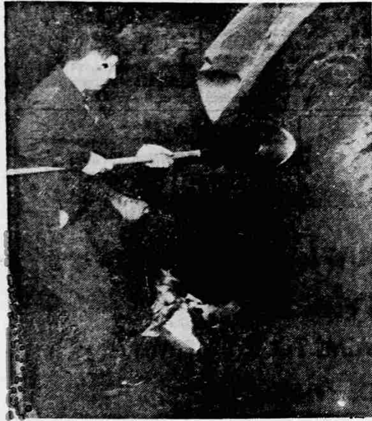
WORKMEN RECOVER BODY —Workmen in Pasadena pull body of Bill Yancey, 47, excavating contractor from cave-in of a sewer excavation which collapsed and buried him. Yancey, a hero in the 1949 Kathy Fiscus tragedy, died a mile and one-half from the spot where he labored 48 hours in the unsuccessful attempt to rescue the little girl from a well.
