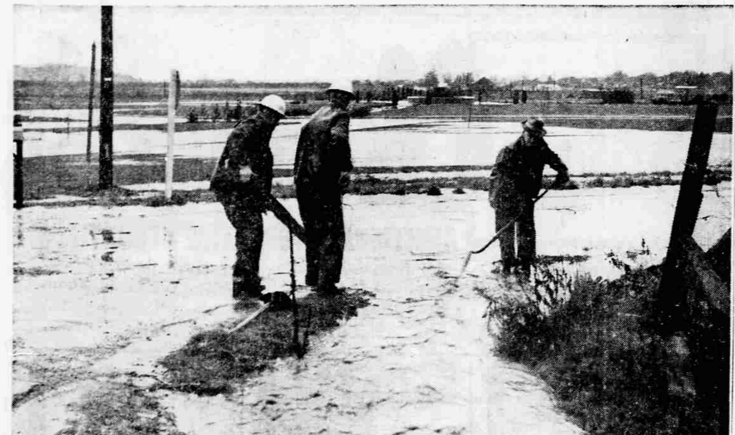
CLEAN CULVERT —As water pours across Bellingier lane at the Arnold lane intersection southwest of Medford, a county road crew removes debris from the upper end of a culvert so water won't run over the roadway. Further up Bellingier lane the water cut away a section of the asphalt paving. Although the high water did quite a bit of damage throughout the county, the worst hit was a section along
