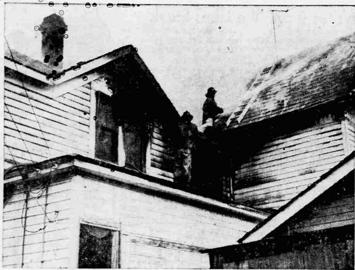
SECOND FLOOR GUTTED —Medford firemen battle flames which gutted the second floor of the two-story Oscar Chinn residence, 1827 North Riverside ave., yesterday afternoon. Firemen said the blaze originated from a defective flue installation in a vacant second-story apartment. Mrs. Clyde Bedington, daughter of the owner, noticed fire in the attic and turned in the alarm about 12:30
