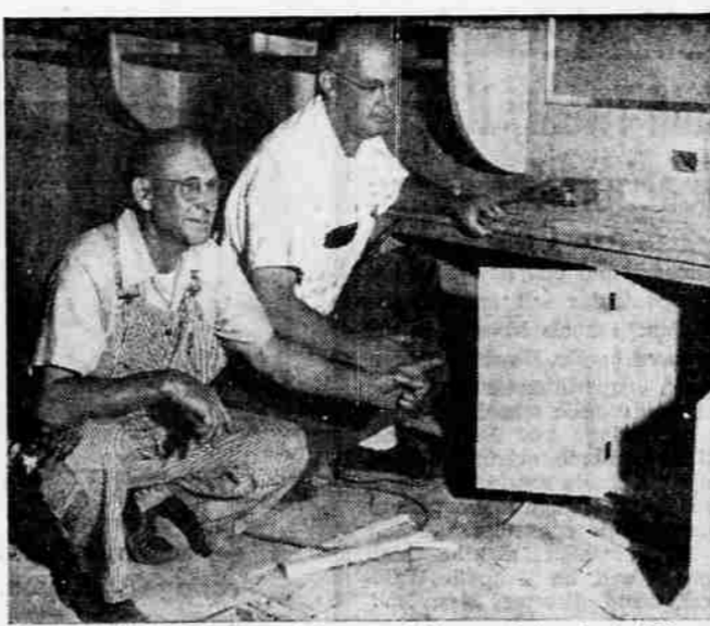
PAY AS YOU GO —Ernest James, right, superintendent of Phoenix schools, consults with Charles Soper, elementary school custodian, on built-in sink units for the new primary addition. Built on a "pay-as-you-go" basis, an additional two primary rooms will be ready for occupancy when school starts.
