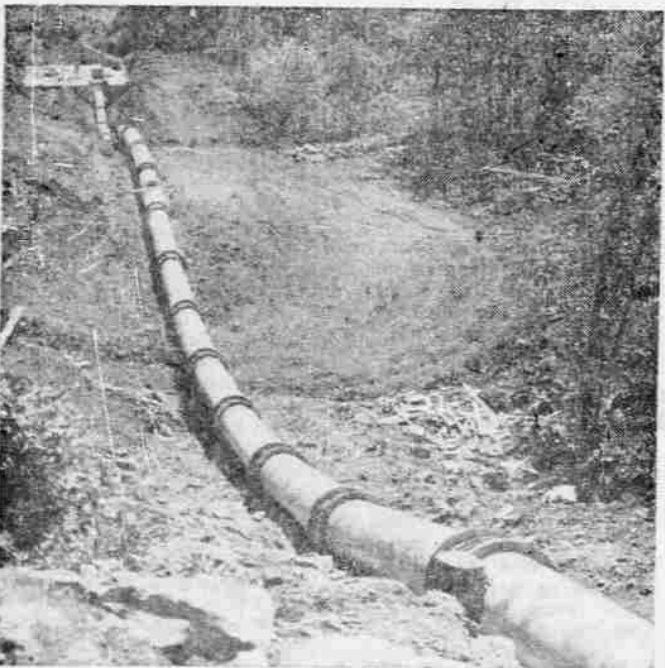
LOWER END OF PENSTOCK —Like a giant snake lying on the steep hillside, the 42-inch steel penstock will carry water to the new generating plant in the Nichols gap area north of Eagle Point. The water will come from an irrigation canal owned by the Eagle Point Irrigation company. Energy from the water had formerly gone to waste as it cascaded down a series of drops to reach distribution laterals at a lower level. Permission to use the water was granted to Copco in exchange for maintenance of the ditch above the site. The water comes from Big Butte creek.
