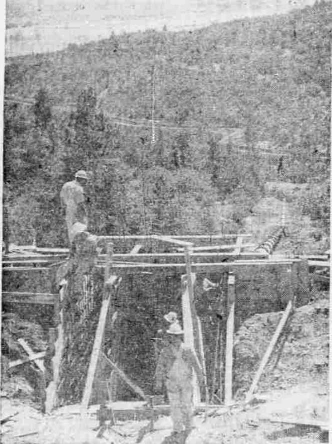
UPPER END OF PENSTOCK —At this point, more than 400 feet higher than the new Eagle Point power plant, water will be collected in a small forebay for its 1,880-foot shoot to the turbine at the bottom. Workmen, above, who are completing forms at the opening of the penstock, had to board up the hole to keep back the gale of hot air that escaped from the pipe during the day. The penstock disappears from sight in the picture where it starts down the hill at a steeper angle.
