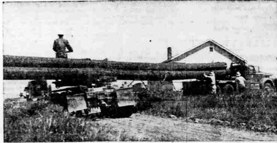
POLE TRANSPORT —A truck and trailer, which has a steering device, carry power poles to the point where they will be raised and set in the ground. The poles support three
