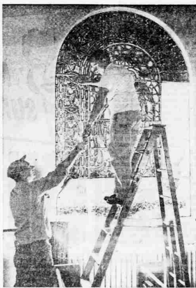
WINDOW INSTALLED —Al Lane (left) and Robert Wickman of the Medford Plate Glass and Mirror company install the stained glass memorial window at the First Methodist church last week. The window, made by the Cummings Studios of San Francisco, is in memory of Mrs. Beulah Faber. It was installed in the large center window of the south wall of the church. Dedication services will be announced later. (Knackstedt photo)
