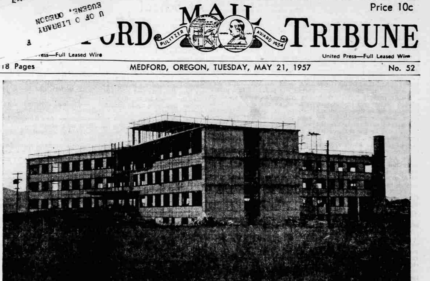
TAKING SHAPE —Construction of the new Rogue Valley Memorial hospital at Barnett and Murphy rds., Medford, is shown in another progressing stage in the above picture. The front of the hospital, which is estimated to cost a total of about
