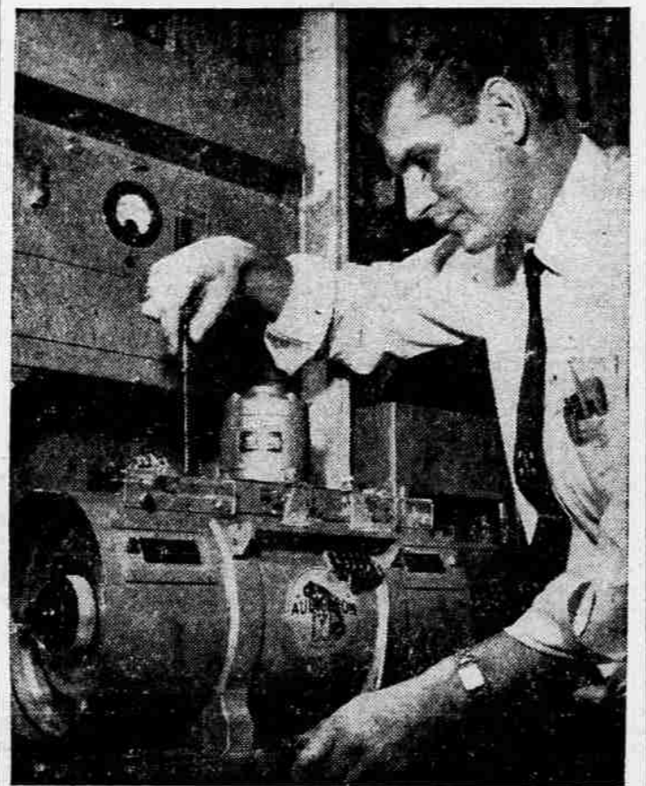
TIME MACHINE—"Audie," one of Pacific Telephone's time machines in Portland, is adjusted by Senior Switchman Stan Boucher. It handles 53,000 calls a day for the correct time.
