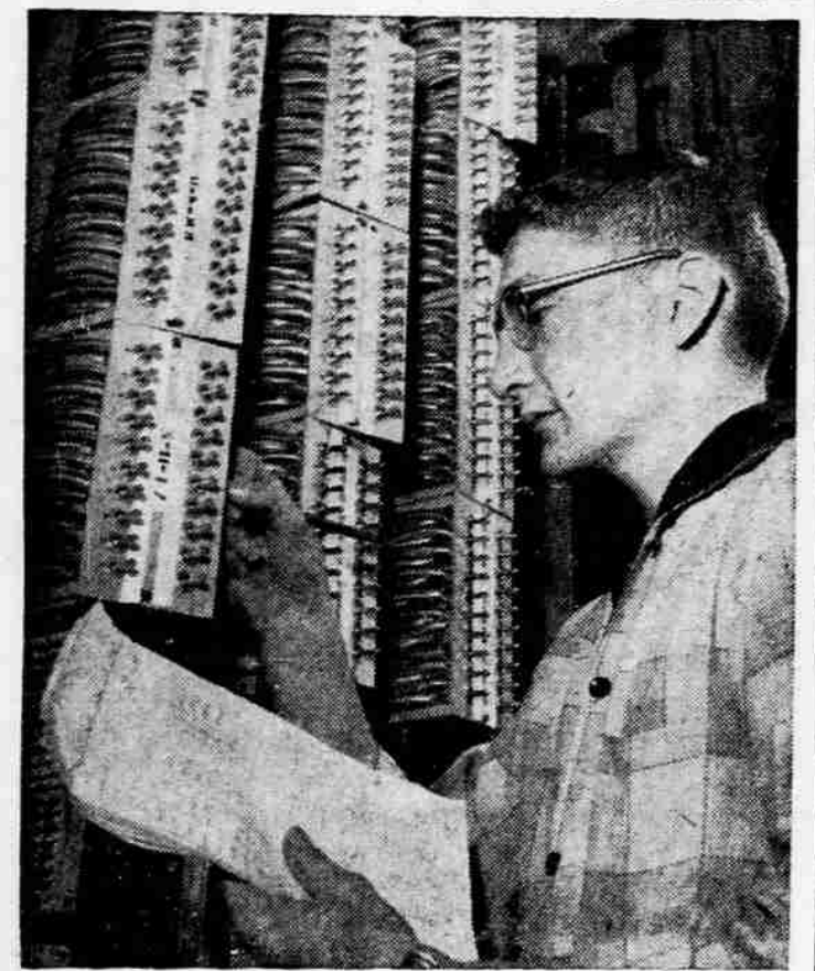
SWITCHES INSPECTED —Switches, shown being inspected here by Bob Lyons, Western Electric employee from Medford, will put life into the new Phoenix-Talent central office when it is placed in service April 27. Pacific Telephone is spending more than $200,000 in establishing the new exchange and introducing KEYstone 5 telephone numbers.
