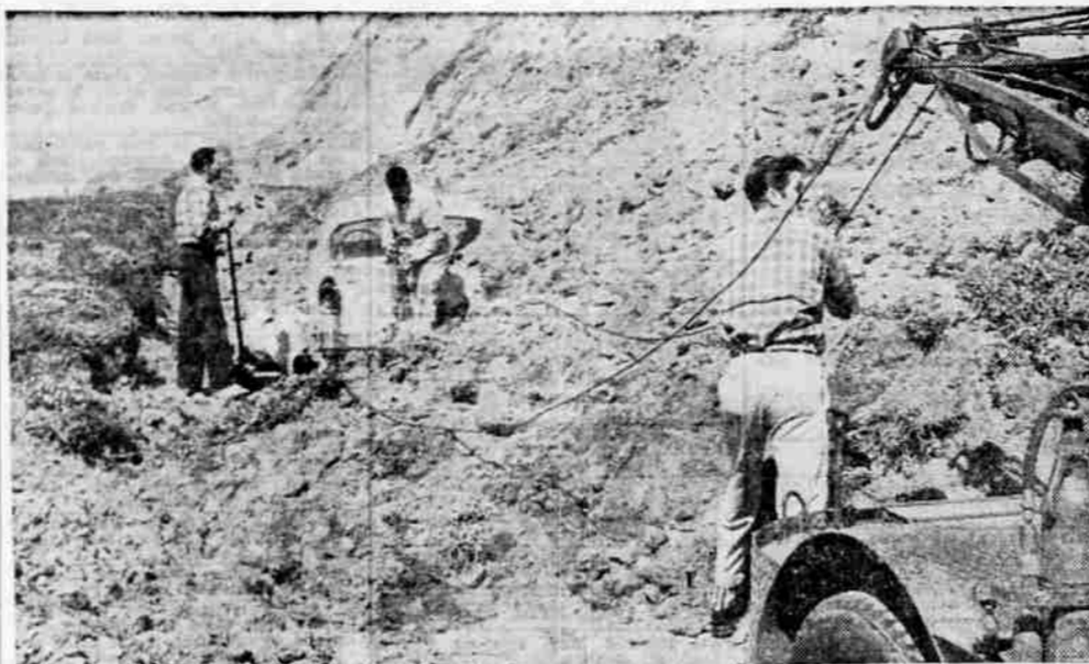
DIGGING OUT —Workmen dig out one of three cars partially buried when sections of the coast highway 10 miles south of San Francisco were covered by landslides caused by earthquakes that hit Northern California. Occupants of the autos suffered only minor injuries and shock. Some sections of highway slid completely away.
