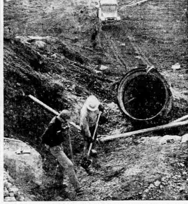
LARGEST MID PROJECT —Medford Irrigation district crews are shown preparing the foundation for two 4 by 14 foot bays that will traffic water from the siphon (at right) during the winter and be used for regulating purposes in the summer. Installation of the 1,860-foot long siphon across the valley floor, about a half mile below Phoenix, has been completed. The siphon damaged by floods with one having a 75-year life expectancy.
