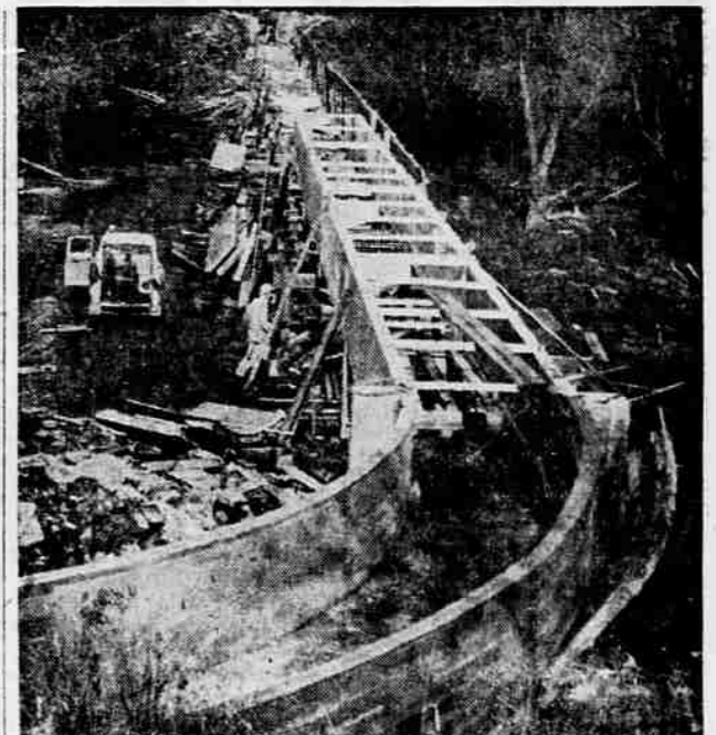
FIRST FLUME OF KIND IN AREA —Above is the flume connecting the main canals of the Rogue Valley Irrigation district, which will serve 90 per cent of the district. Advantages of the $14,500 structure include easier erection in adverse weather and terrain conditions and eliminate trash racks that impede water, which characterized the former design. It is probably the first pre-cast reinforced concrete flume ever built in this area, according to irrigation district officials.
