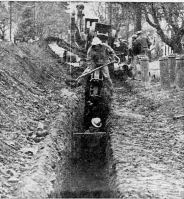
FIFTH STREET TRUNK —The last of three smaller trunk lines was laid last week as workmen were about to finish construction on the $90,000 Phoenix sewer system. Trenching was comparatively easy, according to contractors, since no rock or other obstructions were encountered. One of the things they had to watch for was water pipes beneath the surface of the ground. One is visible near the workman in the trench above. Depth of the trench varied from five to 12 feet.
