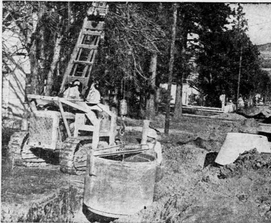
MANHOLE INSTALLATION —Using a large crane mounted on a crawler-type tractor, workmen, above, drop a large section of a pre-cast concrete manhole into place. A concrete foundation will support the heavy unit
