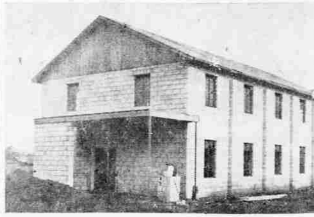
UNDER CONSTRUCTION —Mt. Pitt Avenue Church of the Nazarene educational unit shown above at Mt. Pitt ave. and Chestnut st. is one of the several buildings now under construction by churches in the Medford area. The Mt. Pitt Avenue church, sponsored by the First Church of the Nazarene, will meet in the unit when finished until the other two buildings in the group are completed. The Rev. Dwayne Batchelor is pastor of the congregation.
