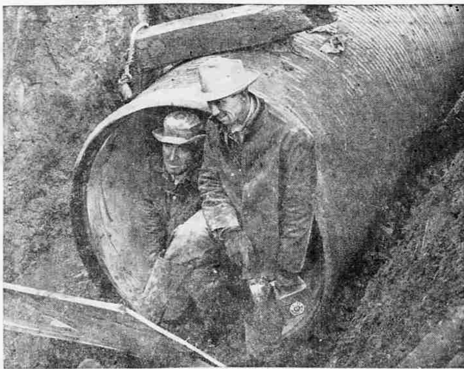
SEAL JOINTS — MID employees, Jim Gibbs and Ralph Kime, come out for a breather after cementing joints inside the 48-inch irrigation tile being laid south of Phoenix. More than 1,200 feet of the tile, in 32-foot sections,
