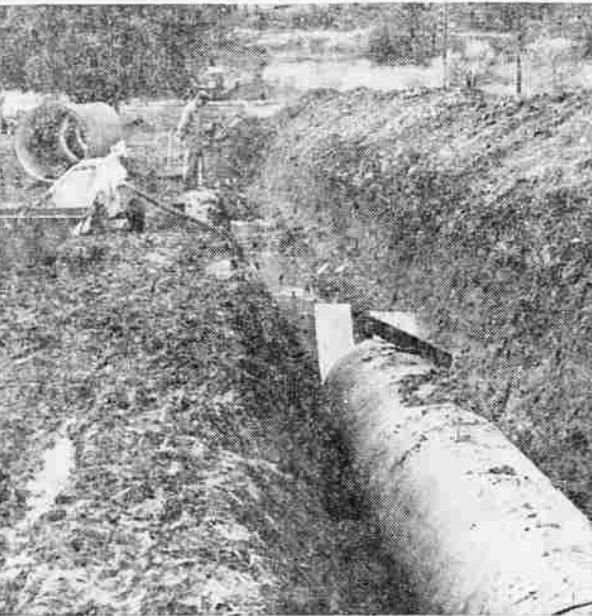
NEW SIPHON — Cement tile, being laid underground instead of on the surface will replace the old wooden siphon south of Phoenix, in use since 1921. The work is being done by the Medford Irrigation district instead of through a contractor, which, according to MID manager, Jack Hoffbuhr, will save the district a considerable amount of money. Nearly all the trenching has been done except for the approaches on either end. Work is expected to be finished well in advance of the coming irrigation season.
