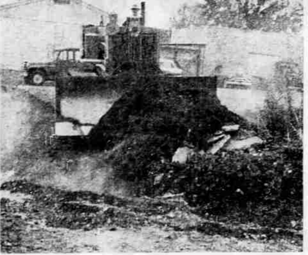
BEAR CREEK BANK WORK —Embankment work on the west bank of Bear creek where the interceptor sewer was washed out in last December's floods, is presently being constructed by F. L. Somers, Medford contractor. Somers was awarded the contract of $19,253 for the work by the Army corps of engineers, Portland. The project includes 5,620 cubic yards of excavation, 500 yards of embankment from gravel borrow and 4,020 cubic yards of dumped stone revetment. All excavation work on the bank has been completed and gravel layers six inches thick are being constructed. A layer of stone from 1 1/2 to three feet thick will top the gravel. A bulldozer is shown above clearing trash from the bank which will be buried under the gravel and stone layers. Work on the project started Aug. 29 and is scheduled to be completed in about two weeks.
