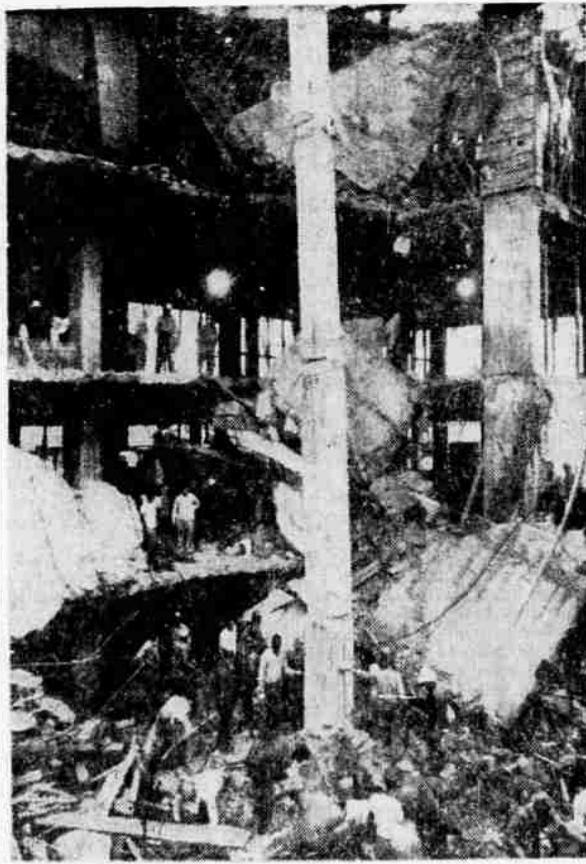
BUILDING COLLAPSE KILLS 10 —Rescue workers (bottom) stand quietly as they listen for possible sounds from trapped men under pile of rubble after this four story building under construction at Jackson, Mich., collapsed. The job superintendent said cranes will have to remove big concrete and steel pieces before shovels can be used to get at the bodies of victims.
